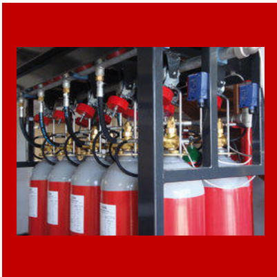
Electrical Panel Gas Flooding System
