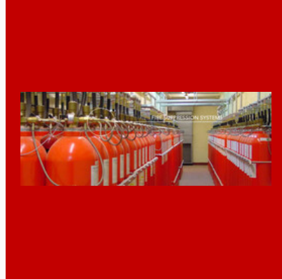
Automatic Fire Suppression System
