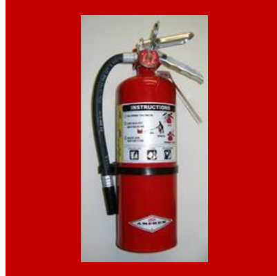
Fire Extinguisher Cylinders
