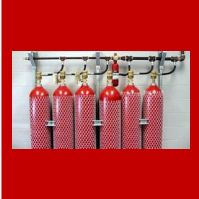
Automatic CO2 Gas Flooding System
